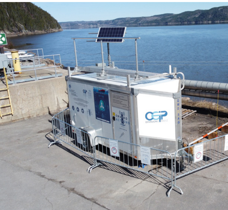
↑ Overview of the real-time data collection station for the Enviro-Actions project led by INREST, located at the marine terminal
